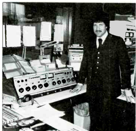
LPB S-20, 10 mixer dual stereo Signature II audio console installed in WGLU air studio.
