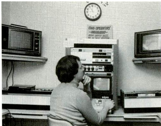
KAKE has four e.j.i. booths and is in the process of building another. The station is also putting in a room for microwave reception
