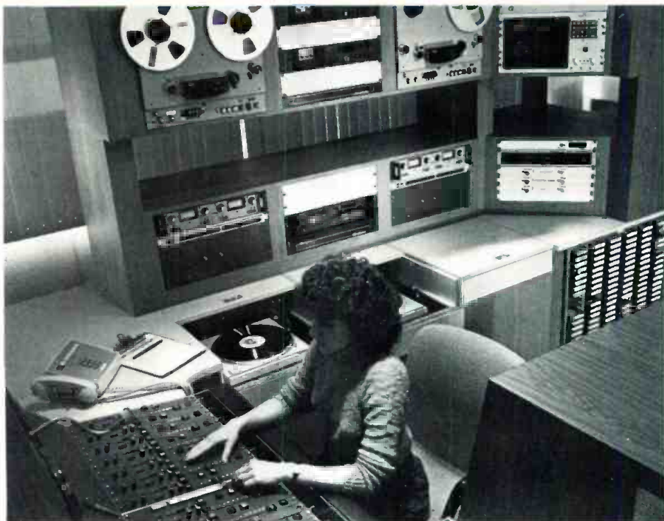
Operating engineer in air control room works on Neve custom console with MCI tape recorders, ITC Delta cart players and Technics turntables in the background.
