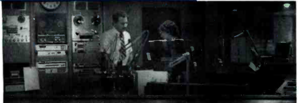
View of the main control and news booth areas as seen from the large studio shows built-in equipment rack (left), accessible from rear.
