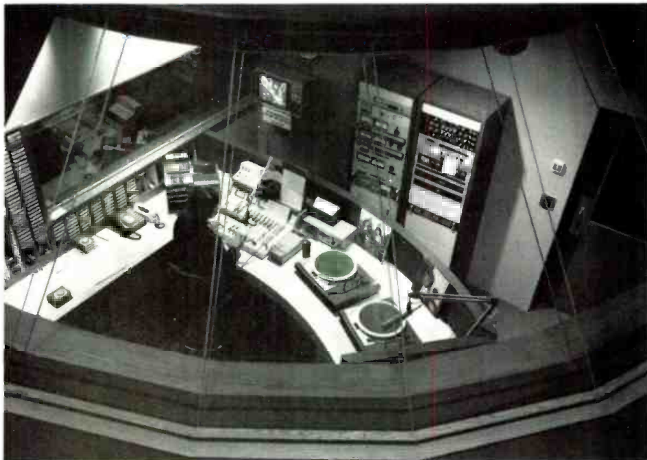
The FM studio is on the opposite side of the wall from the AM in the semi-circular, glass-enclosed air studios, centrally located.
