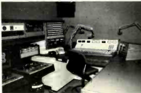
WDBO-AM's production studio is one of three production rooms in the new AM/FM facility.
