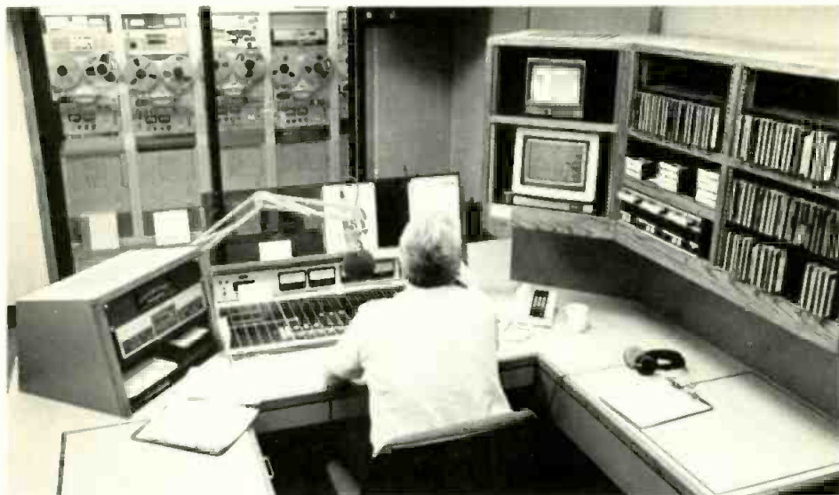
Announcer Bill Norris is able to look into the room, which holds equipment racks from KQXT-FM's on-air studio.
