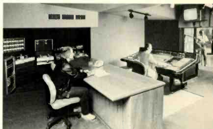
A complete audio recording studio allows full sweetening functions with an SSL 6000E console, Eclipse synchronizer, and Studer multitrack recorders.
