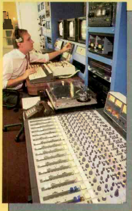
A Sony MXP-2000 console runs the audio in WSYT's production control suite.
