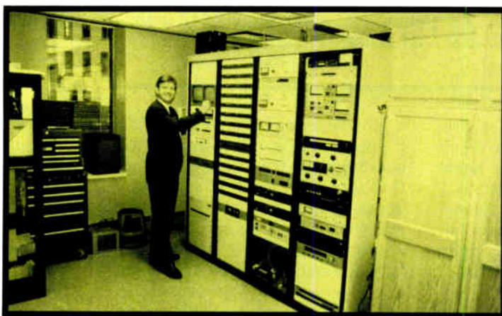
WCUZ's operations manager Bill Ashford adjusts the RPU monitor panel in the facility's tech center.
