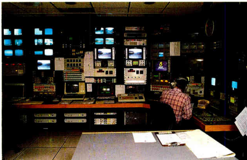
KTLA's John Ferguson watches the helm in the station's transmission control room.
