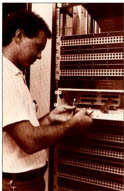
Vista United Telecom engineer Perry Lockhart prepares fiber optic cabling for a Disney-MGM Studios patch panel.
