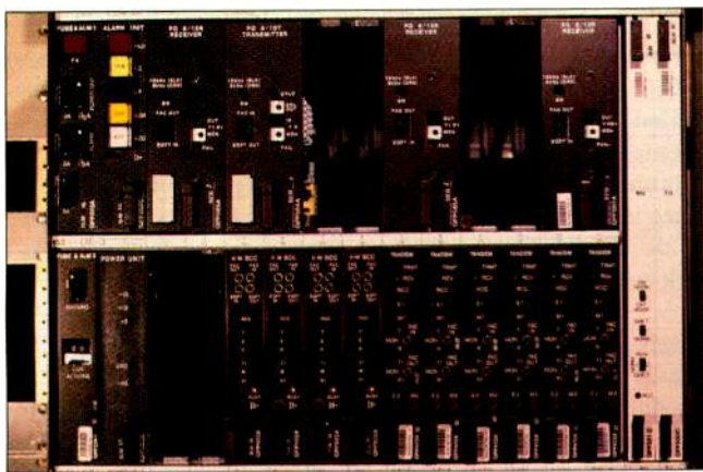
A rack of T-1 hardware. The number and/or types of channels on the T-1 carrier can be reconfigured simply by changing cards in the racks at both ends of the circuit.
