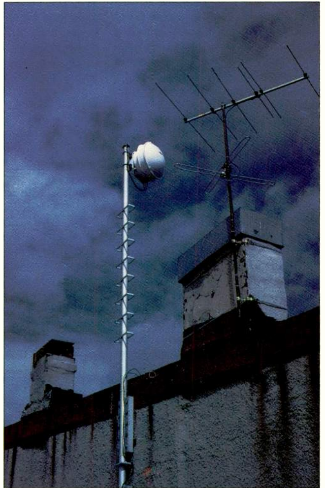
Station-end 23 GHz STL antenna at WJHU-FM, Baltimore, using M/A-COM two-foot dishes. Because of high-rises along line-of-sight path to preferred transmitter site, a 950 MHz STL here would have required substantially higher tower, which was prohibited by zoning laws. Narrower beam width of 23 GHz system allowed use of this lower tower.
