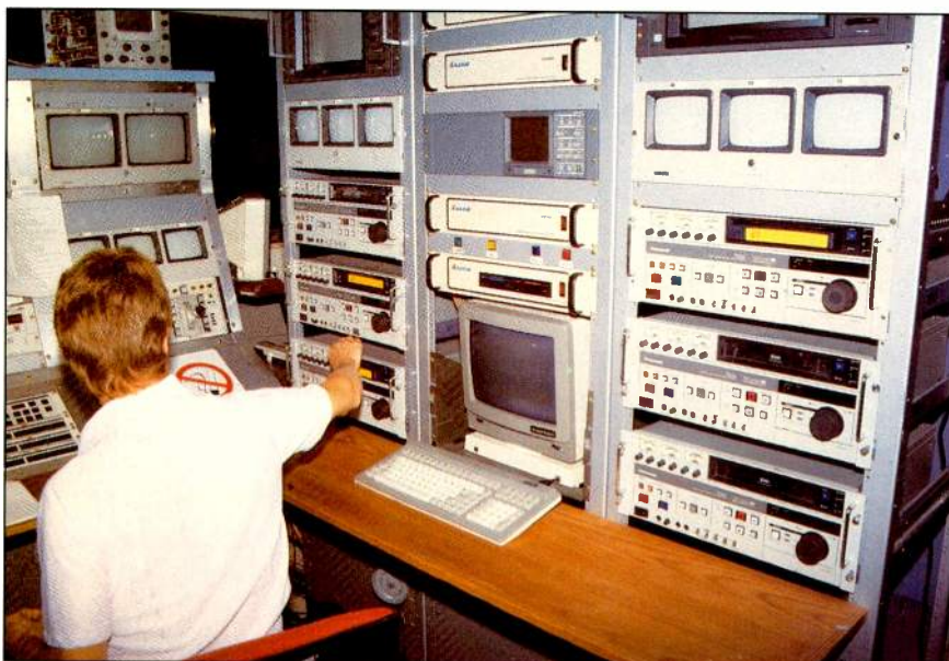
Any one of KCCO/KCCW's seven S-VHS decks (one not shown) can be fed into either of two program lines. Chief engineer Pat Driscoll loads a machine in preparation for spot play.
