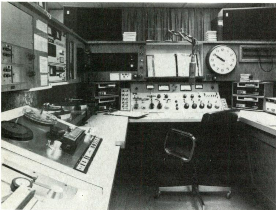
The WFLN horseshoe control room arrangement shown here allows their engineers access to the wiring and equipment. The walk space around the studio furniture is just enough to allow adequate working room. (Photo courtesy of WFLN-AM-FM, Philadelphia)
