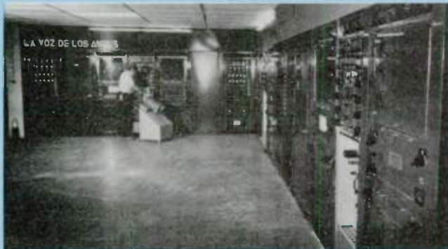
This look inside the HCJB transmitter building shows several RCA BHF-100 100 kW shortwave transmitters.
