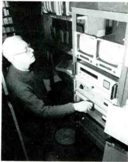
Engineer Bob Sutherland operates the controlling devices for the earth station. The Scientific-Atlanta package will automatically locate and polarize for each satellite which is currently airborne and can be expanded to include future "birds" without additional cost or equipment.
