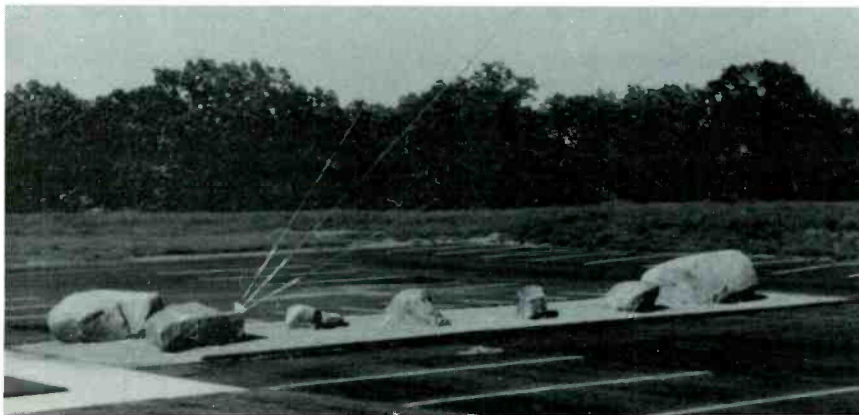
The size of the parking lot required that the building be positioned beneath the guy wires. The ground radials had to be replaced beneath the new parking lots and the building floor slab.
