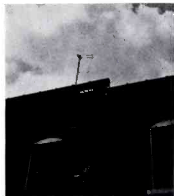
TRANSMISSION LINE FROM RCA VICTOR "TERRA-WAVE" POLICE RADIO TRANSMITTER TO THE ANTENNA AT SPRINGFIELD, MO.
