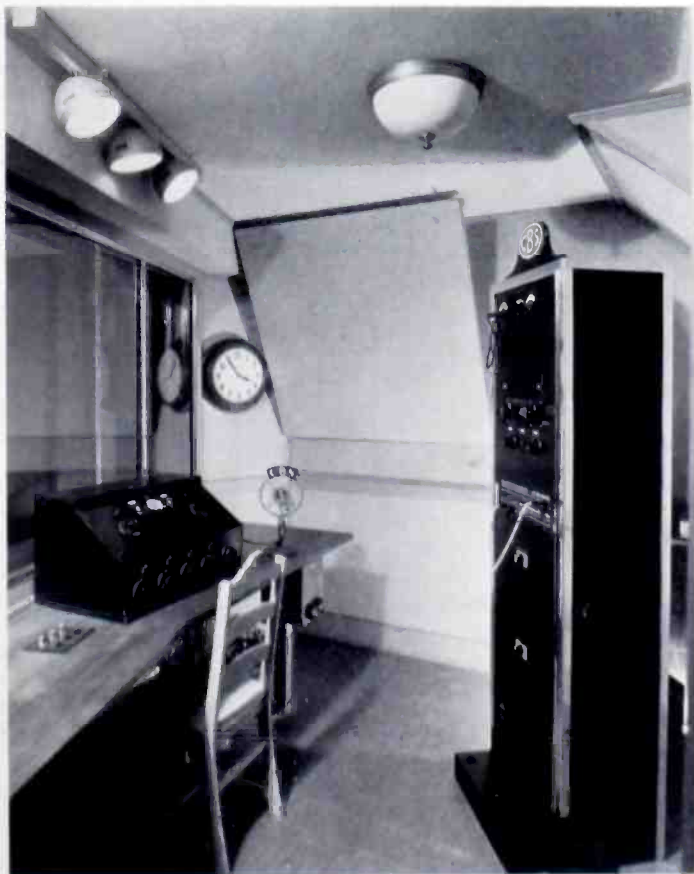
INTERIOR OF COLUMBIA'S NEW CONTROL ROOM AT DETROIT ORCHESTRA HALL— RCA VICTOR EQUIPPED
