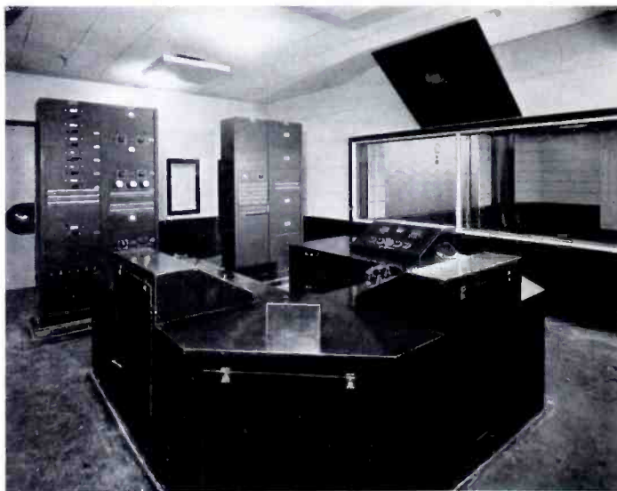
THE COMPLETELY RCA EQUIPPED MASTER CONTROL ROOM AT THE NEW STUDIOS OF WIP
