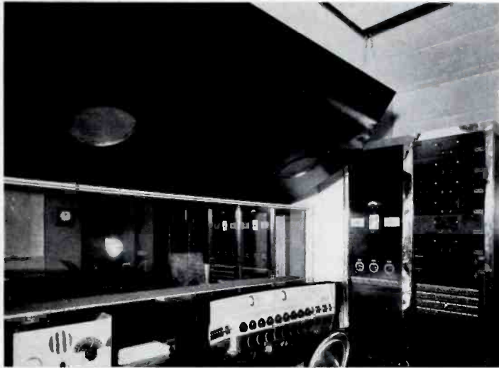
Figure 4. Studio Control Room Equipment.
