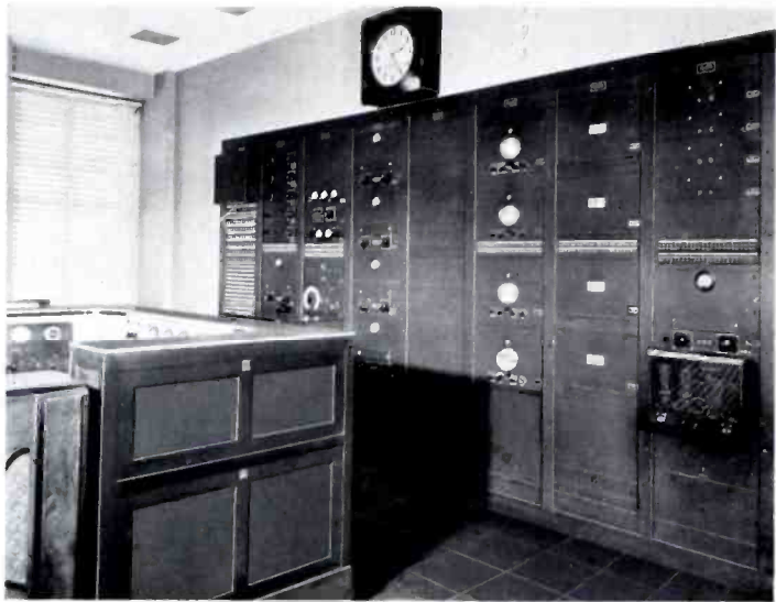
A view of the RCA Speech Input Equipment installation.
