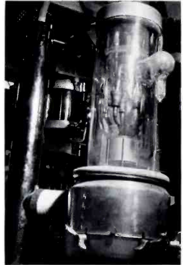
A closeup of a 100 KW tube used in the 50 KW transmitter.
