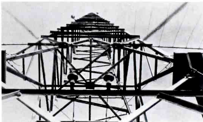
A "shot" from below giving a view of the petticoat insulators and the counterpoise.
