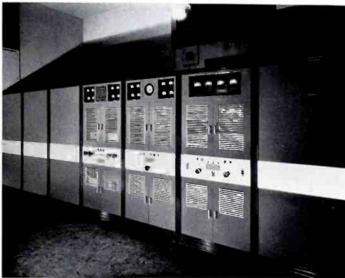
The New RCA 5-C, 5 KW transmitter installed at WFBC.
