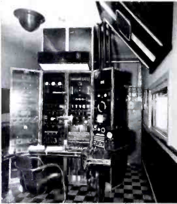
Main control room of WBEN between "A" and "B" studios.
