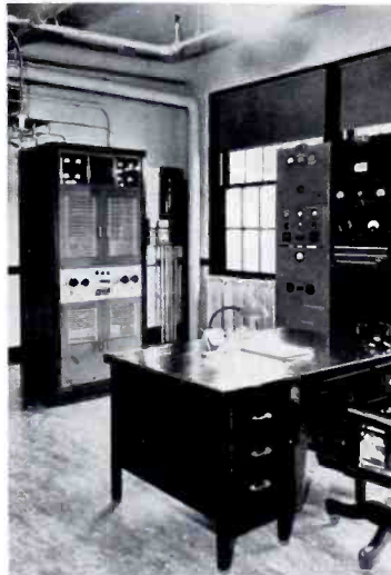
Inside the transmitter house at WEBR showing the main transmitter in the background.
