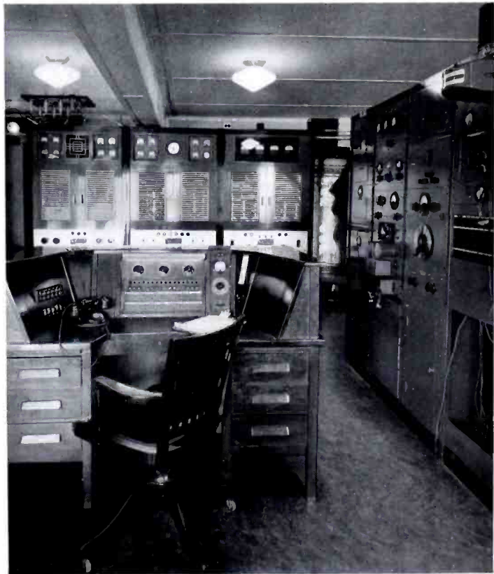
Transmitter house at WBEN, located at Martinsville, N. Y., showing the new 5KW transmitter.
