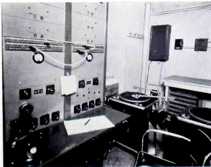
Control room with everything back to normal operating conditions.
