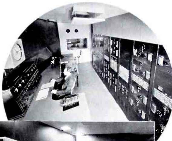
RIGHT: CBS-KSFO Master Control giving a clear view of the equipment racks and outgoing line switching console.
