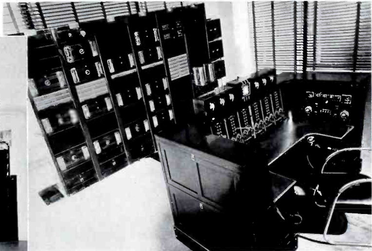
Above: The Master Control Room of WMCA is RCA equipped. This control room is one of the most modern and up-to-date rooms in the country.
