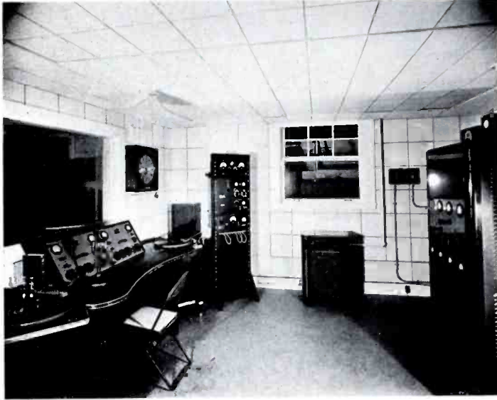
The RCA Equipped Control Room at KBND.
