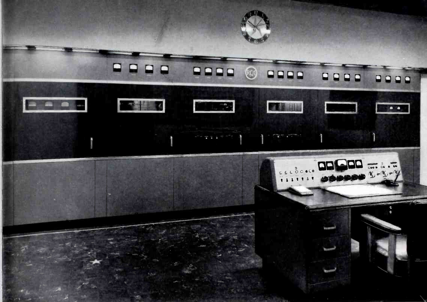
KMPC TRANSMITTER ROOM —The 10-E transmitter, the phasing equipment for the three-tower antenna array, and the speech input and monitoring equipment are all mounted behind the single "unified-front" type enclosure shown above. The operator's console and a monitoring speaker mounted in the ceiling are the only other items of equipment in the transmitter room. The extra panel units which make this ultra-streamlined installation possible are optional accessories with the 5-E and 10-E transmitters.
