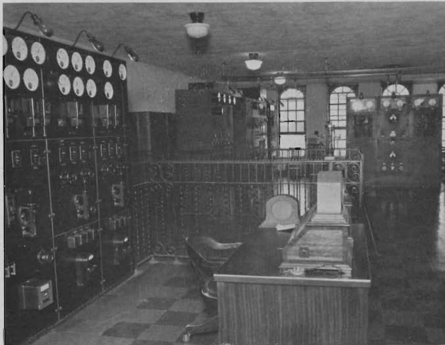
FIGURE 1—RCA 50 K. W. AMPLIFIER, FAR END OF ROOM. 5 K. W. TRANSMITTER AT LEFT END
