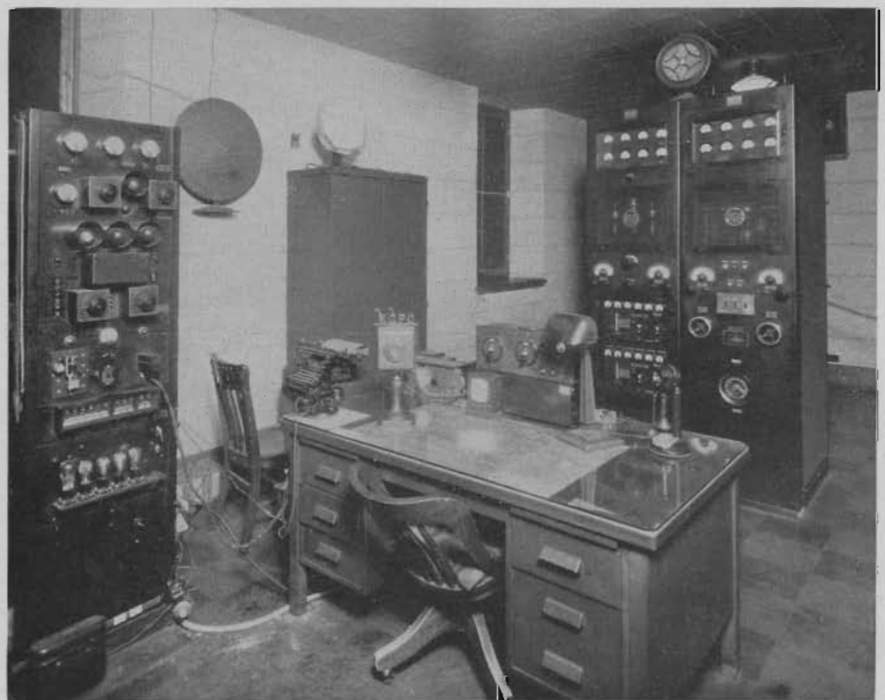
RADIO TRANSMITTER ROOM SHOWING FROM LEFT TO RIGHT SPEECH INPUT, RADIO OPERATOR'S DESK AND RCA TYPE 1-B TRANSMITTER
