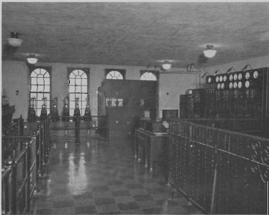
FIGURE 2—NEW RCA RECTIFIER, CENTER PANEL
