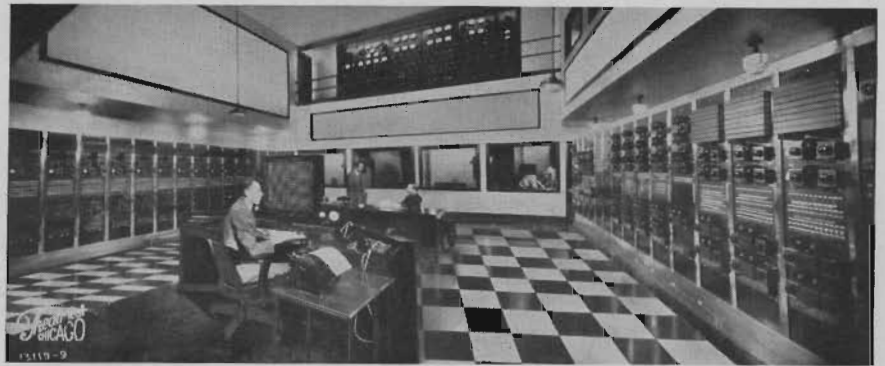
FIGURE 3—MAIN CONTROL ROOM AT NBC CHICAGO STUDIOS. (SEE TEXT)
