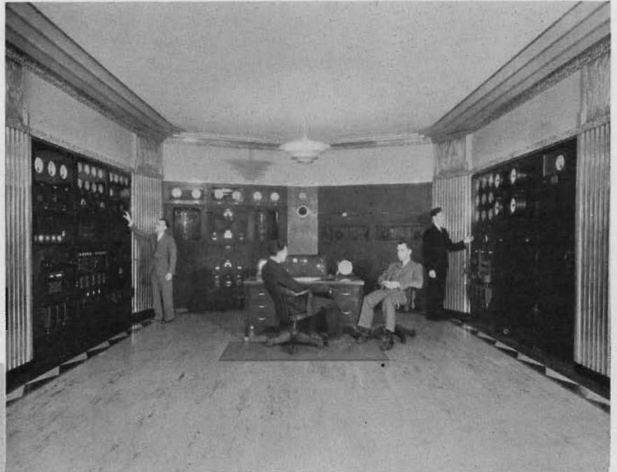
MAIN TRANSMITTER ROOM OF THE NEW WJZ INSTALLATION RECENTLY COMPLETED AT A COST OF $300,000. THE MANNER IN WHICH THE DECORATIONS HAVE BEEN CARRIED OUT REFLECTS THE DEPARTURE OF NBC TRANSMITTER INSTALLATIONS FROM THE CONVENTIONAL POWER HOUSE ATMOSPHERE
