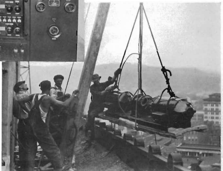
A CRITICAL MOMENT IN THE INSTALLATION OF THE NEW RCA TRANSMITTER AT STATION WWNC IN ASHEVILLE, N. C.
