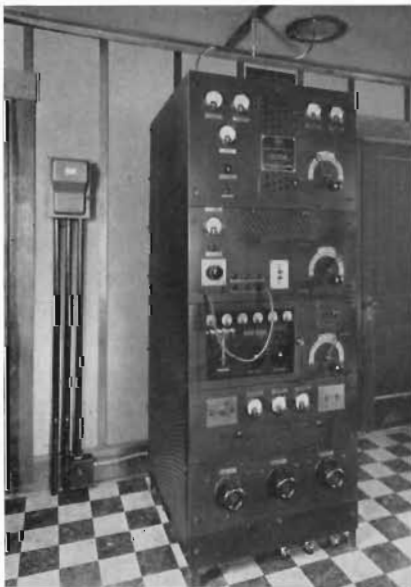
TRANSMITTER AT WORC
