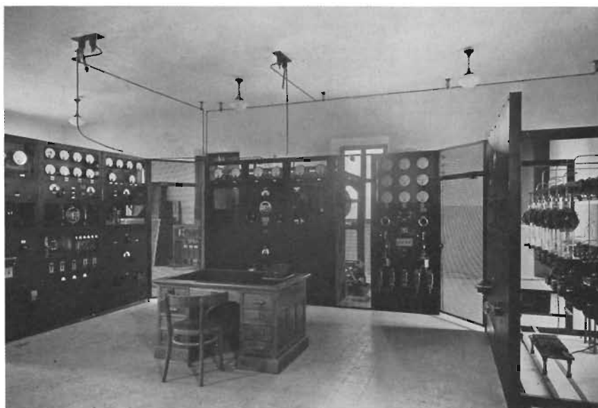
TRANSMITTER CONTROL ROOM OF THE STATION AT ROME, ITALY
