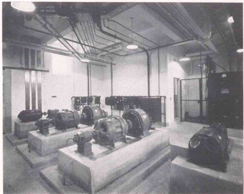
POWER ROOM WBT
