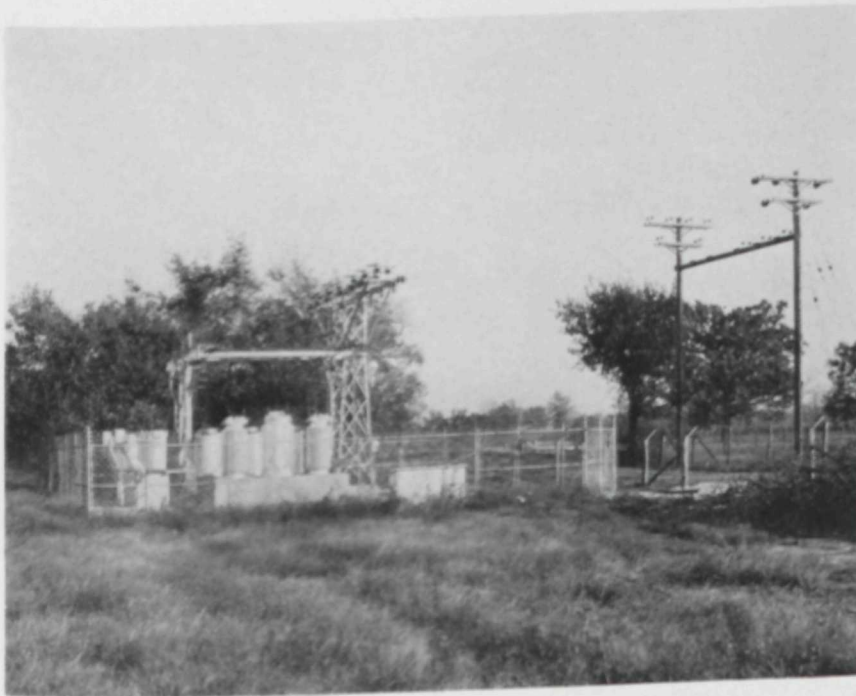
OUTDOOR SUBSTATION AT WSM
