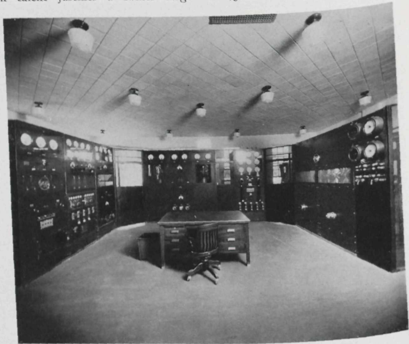
TRANSMITTER ROOM OF THE NEW WSM STATION
