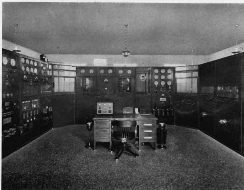
MAIN TRANSMITTER ROOM OF THE NEW RCA 50 K-W STATION FOR WOC-WHO,
