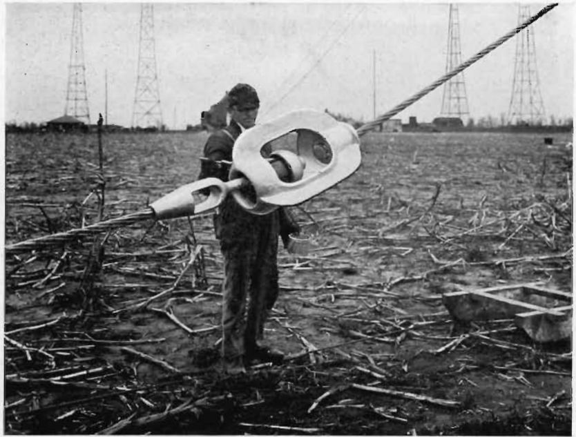
UNIQUE GATHERING OF RADIO BROADCAST TRANSMITTERS. IN THE FOREGROUND IS A SECTIONALIZING INSULATOR IN ONE OF THE GUY WIRES ON THE NEW WLW 500 KW TRANSMITTER TOWER. IN THE BACKGROUND AT THE LEFT MAY BE SEEN THE TOWERS OF WSAI, IN THE CENTER MAY BE SEEN THE SMALL MAST OF THE SHORT WAVE STATION W3XAL, AND AT THE RIGHT MAY BE SEEN THE LARGE STEEL TOWERS OF WLW. RADIATION FROM THE TOWERS OF THE STATIONS SHOWN IN THE BACKGROUND OF THIS PICTURE CAUSED SOME SURPRISING RESULTS DURING THE CONSTRUCTION OF THE NEW TOWER IN THE FOREGROUND.
