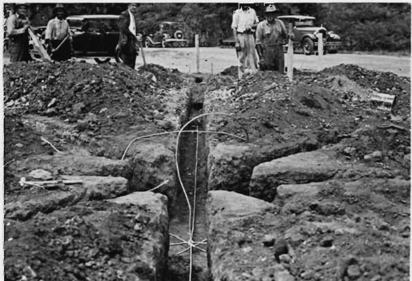
PROGRESS VIEW DURING THE CONSTRUCTION OF THE GROUNDING SYSTEM AT WPET . THE No. 0 STRANDED COPPER CABLE USED IN THIS NETWORK IS WELL BRAZED AT ALL JOINTS.
