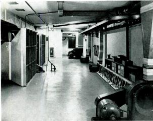
FIG. 7. Air plenum chamber. Six high velocity blowers draw air from this basement room and circulate it throughout the driver and amplifier cubicles overhead.
