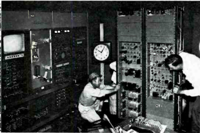
10:06 A.M. Last of the equipment racks are being set in place over trenches in the TV Tape area. The complete color tape recording facility includes (left to right) operations center (3 racks), color processing equipment (1 rack), auxiliary and newer equipment (2 racks).
