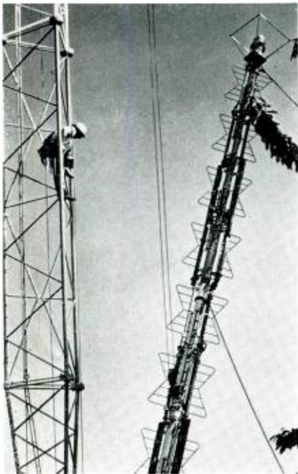
FIG. 3. Custom antenna, Type TF-8AH, about to be lifted to the top of the KGW-TV tower. In normal operation the upper four batwing sections function as the visual antenna, and the lower four as the aural antenna. Each antenna is fed by two 3 1/2-inch transmission lines from a power dividing tee at the top of the tower.
