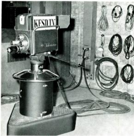
FIG. 5. Camera, intercom, and microphone outlets in Studio 1. To the right are storage hooks for intercom and cable equipment.
