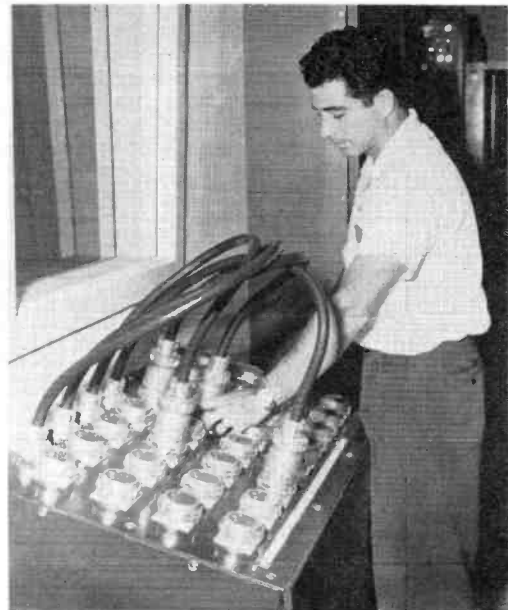
FIG. 11. Camera patch panel enables any camera outlet in the studios, or out of doors, to be quickly patched into camera control equipment.
