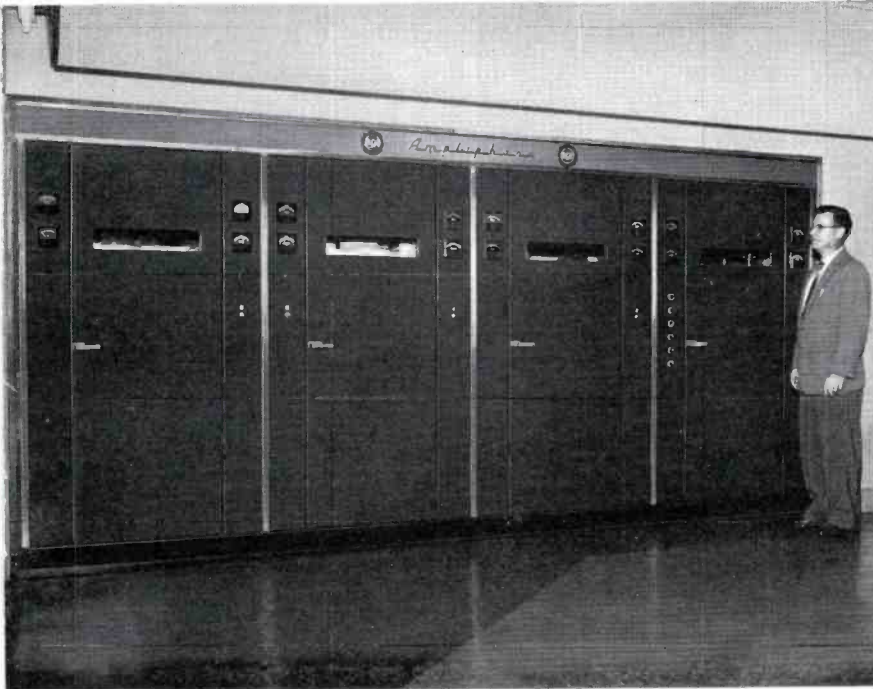
FIG. 3. John Henninger, Chief Engineer of WIBG, at the Ampliphase 50-kw transmitter. The 15-foot wide transmitter has been mounted flush with the wall to produce an attractive easy to maintain installation.
