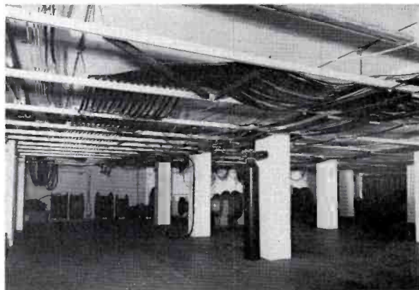
FIG. 6. The wiring vault beneath master control. Utilizing the 5-foot elevation of master control room, the suspension of a power-strut grid permits easy addition or removal of cables and video lines, without disturbing existing wiring. Note the absence of cable trays or raceways. Ten-inch holes under each piece of equipment provides cable access and permits exhausting of filtered, cool studio air through equipment racks.
