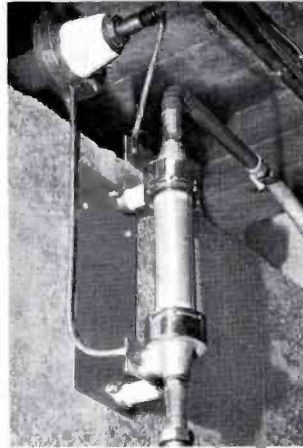
FIG. 11. The wire wound 50-kw dummy load is mounted in the basement just below the transmitters. This unit is capable of dissipating full power generated by the 50-KW Ampliphase Transmitter at 100 percent modulation. A flow of only 15 gallons per minute of ordinary tap water are required for complete cooling of the load.
