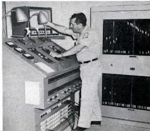
FIG. 11. Tony Maggiore, supervisor of camera and lighting is shown operating the Aerial-Davis lighting board located in production control. Panel to right is Quick Connect Board which can handle 120 20-amp. circuits with no patch cords. Sloping panel to left has 21 dimming circuits. Circuit breakers and transferswitches are directly below dimmers and 72 50-amp. patch circuits are here at knee height. Total capacity of equipment is 200 kw.
