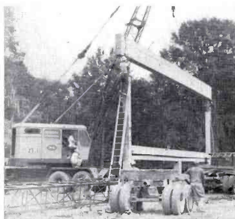
FIG. 26. Installing the first of four 14-ton prestressed concrete beams, which allowed an unobstructed floor area of 50 by 60 ft. In spite of inclement weather the prestressed concrete building was assembled in three days.
