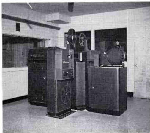
FIG. 7. Projection room with two TP-6CC Film Projectors, a TP-7 Slide Projector, a TP-15 Multiplexer, a 1-V Vidicon Film Camera and a 3-VColor Film Camera. Space left for a duplicate of this set-up is now in process of having equipment installed. (Access holes in floor for this expansion were plugged at the time that this picture was taken).
