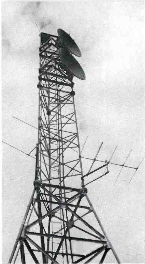
FIG. 15. Tower atop studio building shows mounts for microwave dishes, (also receiving antennas for office monitoring system). This tower is 67 feet high. (90 feet above street or sea level).
