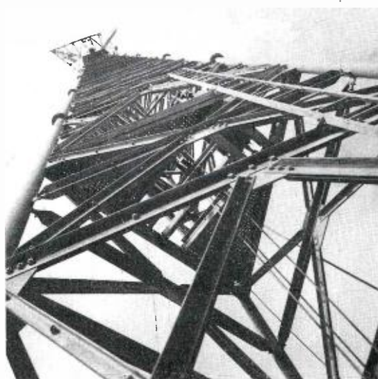
FIG. 4. The solid steel legs of the tower are shown here. Extra strength is obtained from the elaborate cross bracing in the tower. Note that when this photograph was taken the platform erection was in progress.
