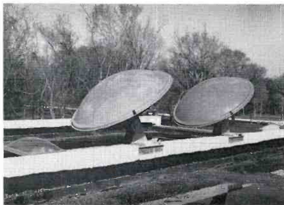
FIG. 17. Front view of microwave dishes mounted on roof of transmitter building. (Note protective plastic covers on dishes).
