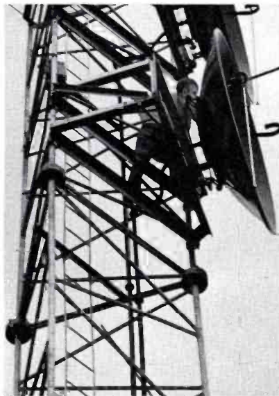
FIG. 22. Engineer lining up microwave dish by means of sighting tube placed on top of it.
