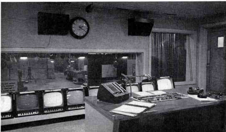
FIG. 8. Production control room. Elevated 5 feet above the studio floor, the director utilizes a row of TM-7 Monitors for program sources. The lighting control board (described elsewhere) is to the right of the switching desk, and the announce booth to the left. Three systems of intercom are available to the director: the push button type which includes the lounge, property storage and announcer's office as well as operating areas, the microphone ceiling speaker system and the standard headset type. (The latter two are tied together). This method of operation with the video and audio control personnel separated from the director has proven very satisfactory.
