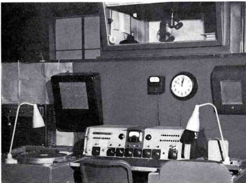
FIG. 12. WTOP originates its all-night show from this small announce booth at the transmitter building. The series 76 console and two turntables are all the studio equipment needed. Normal sound isolation, used in the booth, is sufficient to make room noise from the transmitters inaudible.
