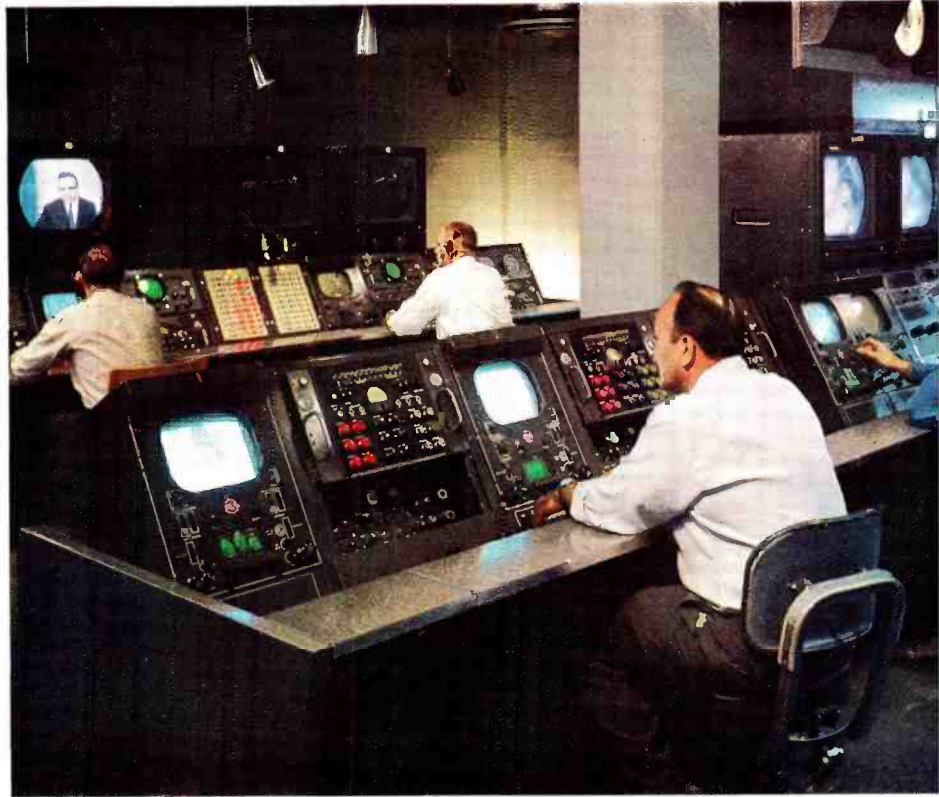
FIG. 2. Master and camera control areas are grouped for production efficiency. Control positions for all four color cameras face a line of color monitors at the front of the room. Master control with its custom built TS-40 Switcher is shown at the right.
