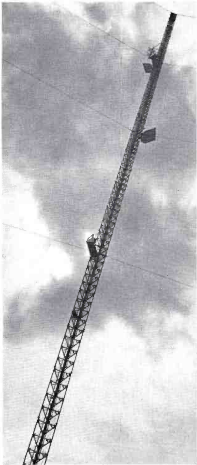
FIG. 16. Tower before erection of big antenna. A 2-bay standby antenna and microwave screens are already in place.
