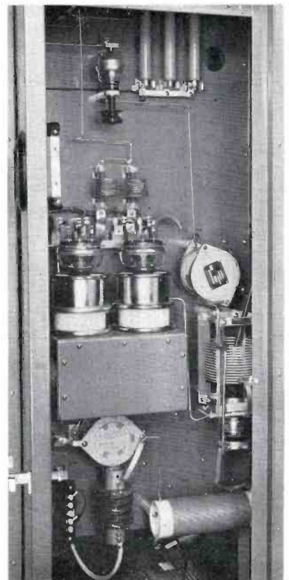
FIG. 10. Full-length photo of PA cabinet. Note the accessibility to all components.
