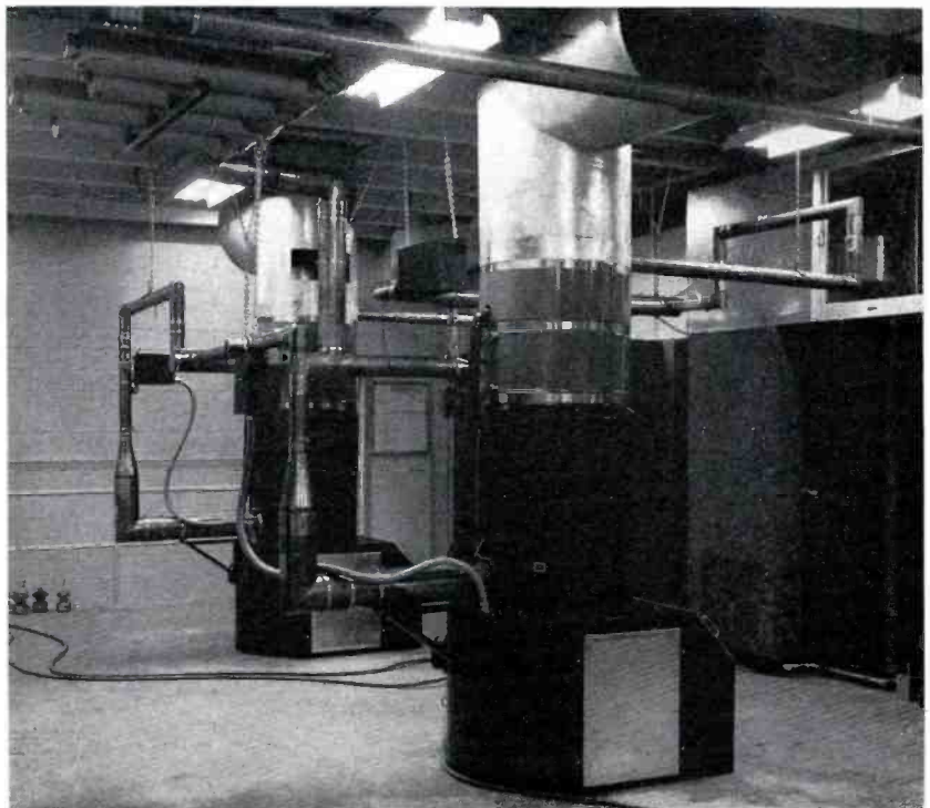
▼ FIG. 7. View of FM transmission line and diplexing equipment. Note that air filters in base of amplifier cabinets have been replaced with sheet metal since cooling air enters cabinet through floor from blower unit in basement. Rear of BTF-10D transmitter appears at far right.
