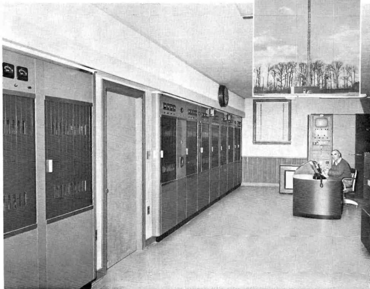
FIG. 1. WBOC-TV's TTU-12A Transmitter as it appears to day. The 600-foot tower and antenna are shown in the inset.
