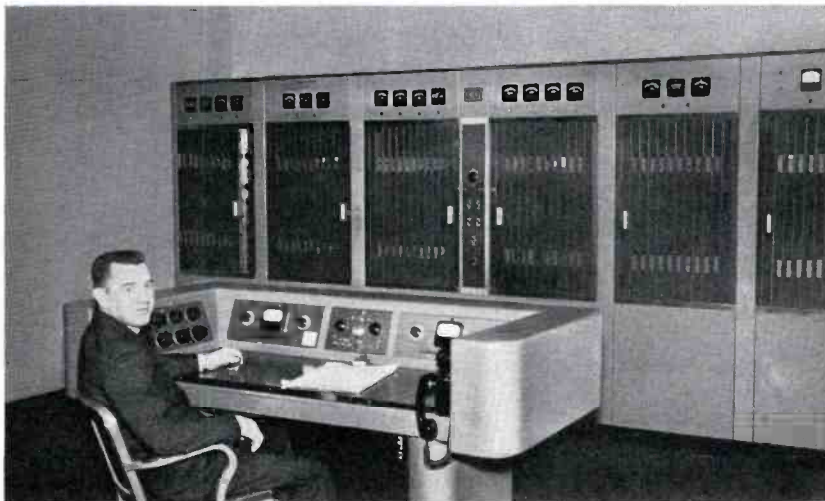
FIG. 10. The AM-transmitter facility. The cabinet at the far left houses the 1-kw (BTA-1M) nighttime transmitter and the next four house the 5-kw (BTA-5H) daytime transmitter. Cabinet at far right contains the antenna-phasing equipment. Transmitter Supervisor Roy Horsman at the console.
