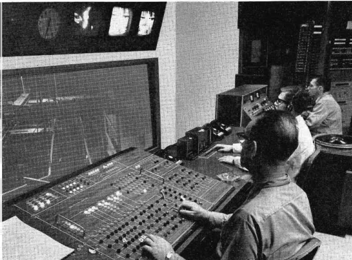
FIG. 15. Control room for Studio One. The control for Studio Two is identical in every respect.
