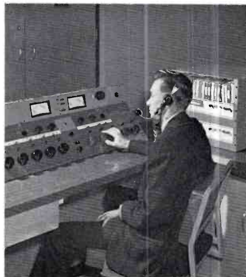
FIG. 30. One of three BC-7 transistorized audio consolettes in new WOC. This is sub-control B. Included are two cartridge tape units and turntable.
