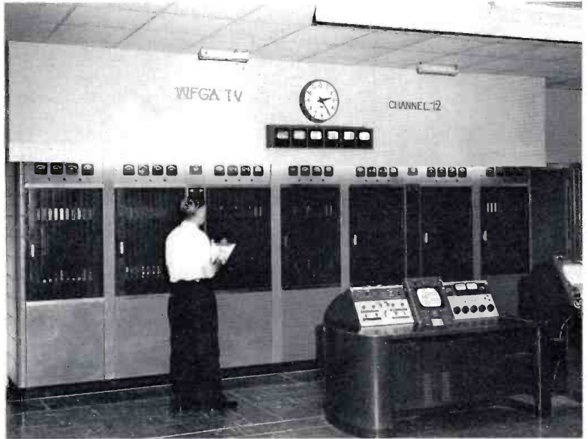
FIG. 24. Type TT-50AH 50-KW TV Transmitter is located in master control room, along with the video control desk and master control switching. It feeds a TF-12BH antenna located behind the studio building on a 922-foot Ideco Tower. The overall height is 996 feet above ground.
