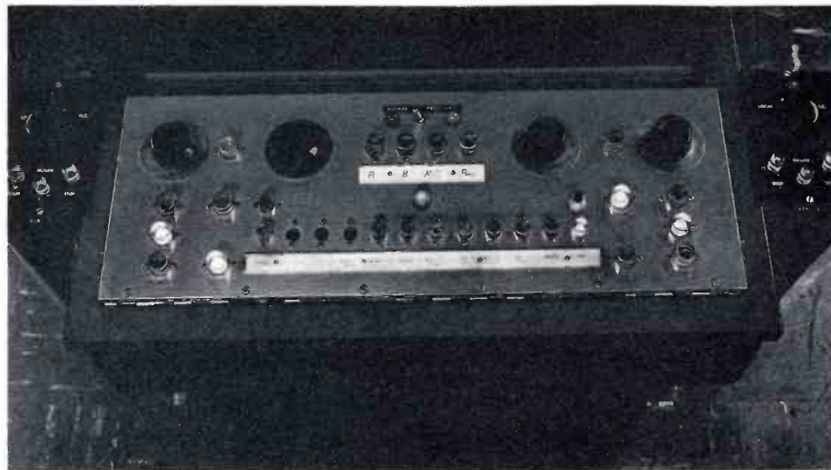
FIG. 20. This is the Projectionist's Master Control Switcher. It controls two TR-22 TV tape recorders, two 3-V color chains, network, remotes and two slide projectors. This overrides every control position except Master Control. It is also tied in with the interlock system of video and audio sources.
