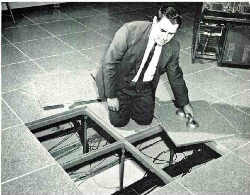
EASY ACCESS TO CABLING is a construction feature of the equipment room floor. A platform floor is elevated two feet above the floor level of Studios A and B. The photo above shows detail of its construction. A strut-like steel framework is supported at intersections by pipe stanchions (threaded for level adjustment). Over this frame are laid two-foot square blocks. The blocks are fabricated of \frac{3}{4} -inch plywood and steel sheets, topped with vinyl flooring, and encased in a frame of thin aluminum. Here a suction cup device (such as that used for handling large sections of plate glass) is being used to lift out the blocks for checking wiring between tape and film areas and the control console. These blocks form the entire equipment room floor. Use of this technique substantially expedited the initial installation of equipment. It also holds promise for ease of maintenance and simplified future expansion.
