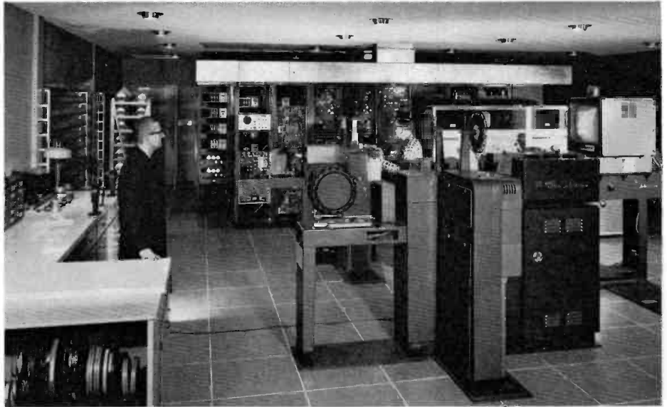
SPACIOUS EQUIPMENT ROOM. Film, tape, and rack mounted equipments are all located in the master control room. This is a view of master control looking from the equipment control console toward the rear of the room.
