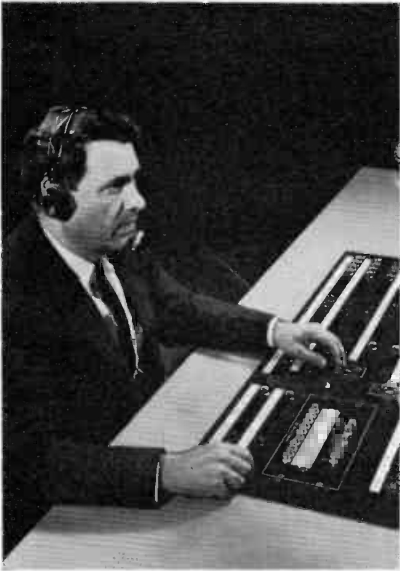
MASTER SWITCHER. This single TS-40 video switching system handles all program switching requirements. It is fully equipped for a multitude of electronic special effects.
