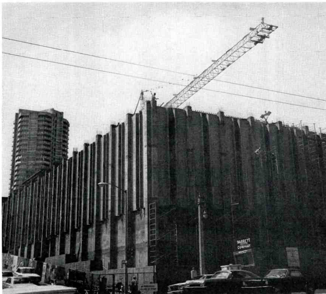
FIG. 21. This shows the KRON-TV building during the construction phase. The nature of the location can be seen by noting the sharp incline of the street. The front entrance is at first-floor level. An entrance halfway back along the side is at second-floor level. An entrance at the rear is at third-floor level.
