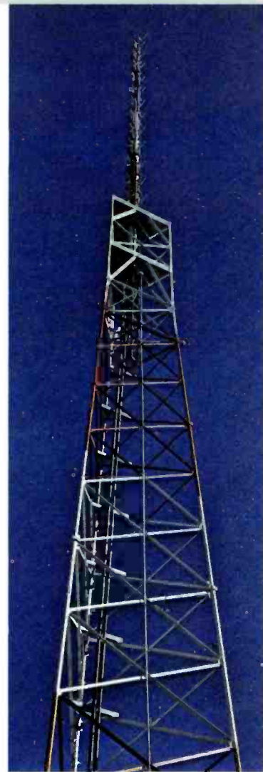
FIG. 15 The TF-12AH superturndstile antenna tops the 100-foot tower on Black Mountain—1220 feet above average terrain. This is also the site of KHBV, the Channel 5 commercial station.
