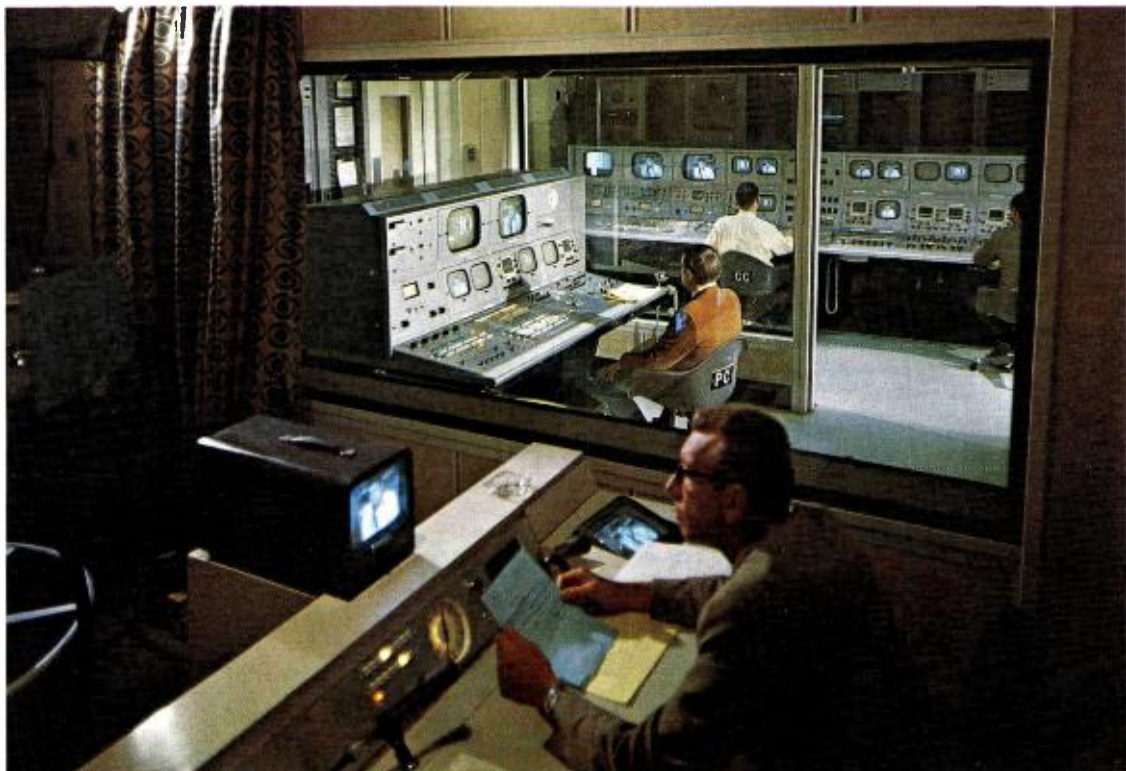
FIG. 12 Announce booth—note visual contact between announce booth, Production Control and Central Control.
