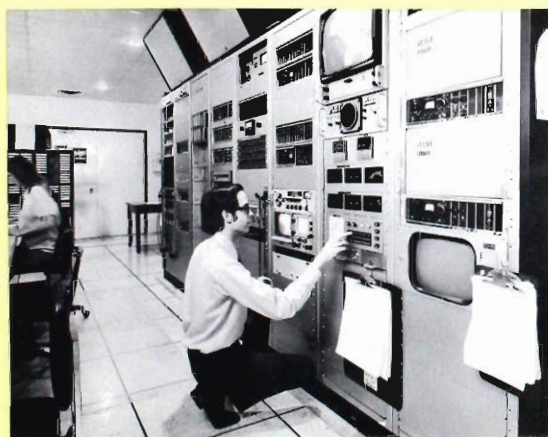
Remote controls for transmitter and microwave system are rack-mounted behind camera control position of console.
