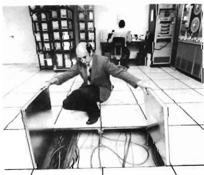
Computer-type flooring under master control room provides easy access to wiring for maintenance.
