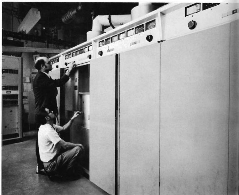
TTU-60, 60 kW transmitter for TV-26 is centrally located on the 50th floor of One Shell Plaza.
