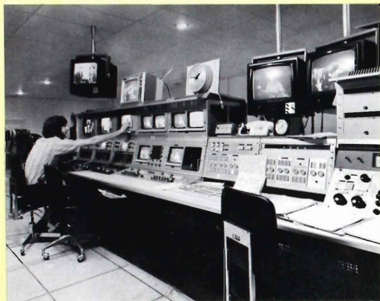
Efficient console arrangement permits simultaneous handling of on-air assignments as well as studio production.
