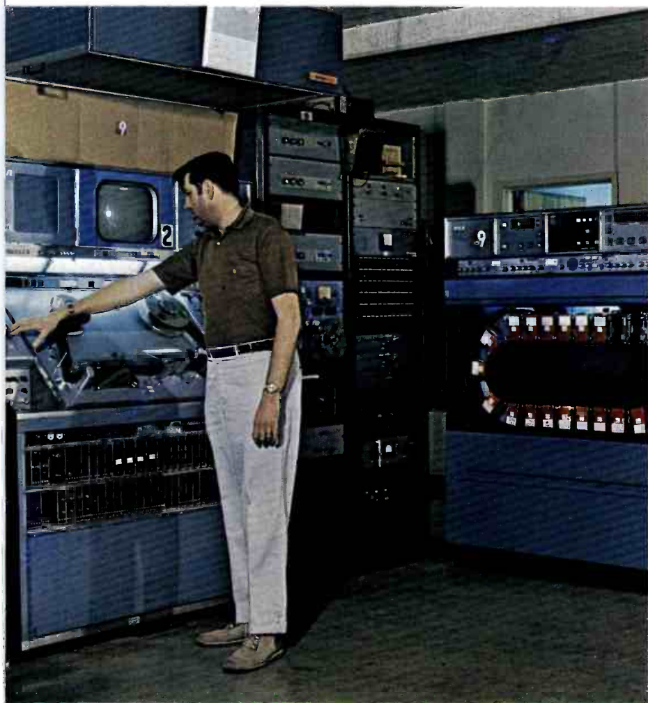
In a switch of roles, WTVC makes use of the TCR-100 as a "master" for making multiple dubs to the TR-70.
