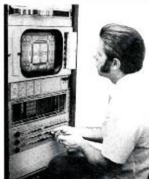
Modules and auxiliary set-up control panel for TK-28 at TAV are rack-mounted directly behind the video operator's console.
