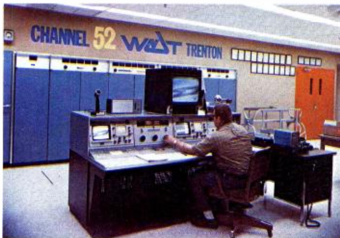
A TTU-60, 60 kW UHF transmitter is installed at each of the four statewide NJPB transmitting locations. The WNJT-TV, Ch. 52, Trenton facility illustrated is typical.
