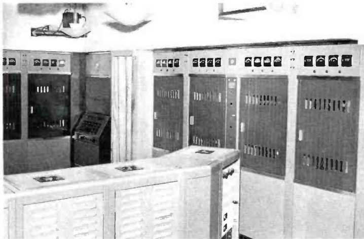
Amplifier cabinets for TT-50AH system occupy much of transmitter room area.
