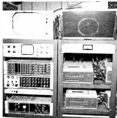
Closeup of equipment racks. Audio system stores in portable cases.
