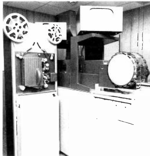
Four-input, two-output telecine system uses a minimum of floor space. Both TK-28 cameras are mounted inboard.
