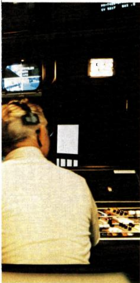
Production studios at KSTW are fully equipped and professionally staffed for commercial production.
