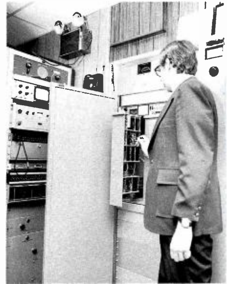
Chief Engineer Larry Vehorn checks TTUE-4A solid state exciter added to upgrade the station's transmission facilities.
