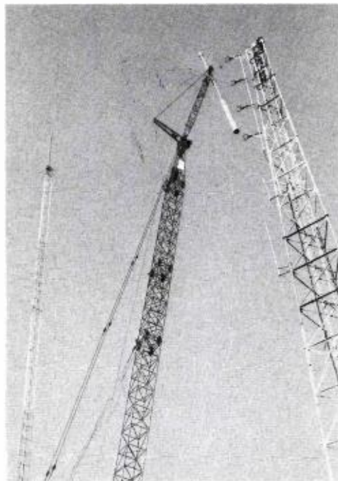
TFU Antenna comes down from old tower for return to RCA for refurbishing and modification.
