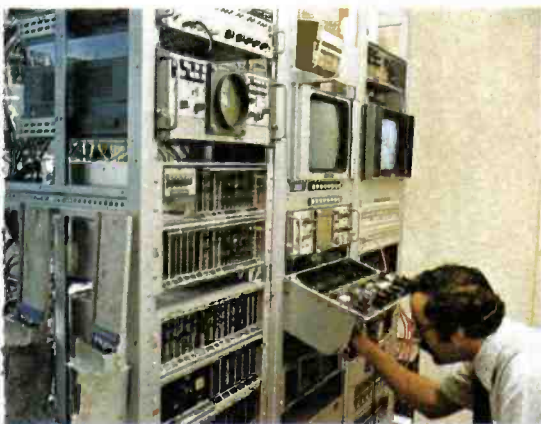
Distribution, monitoring and microwave racks are housed in the Master Control Room.
