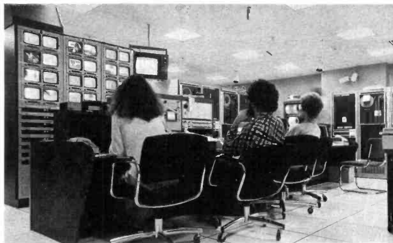
QUBE Master Control houses all video monitors. Also, note computers in background.
