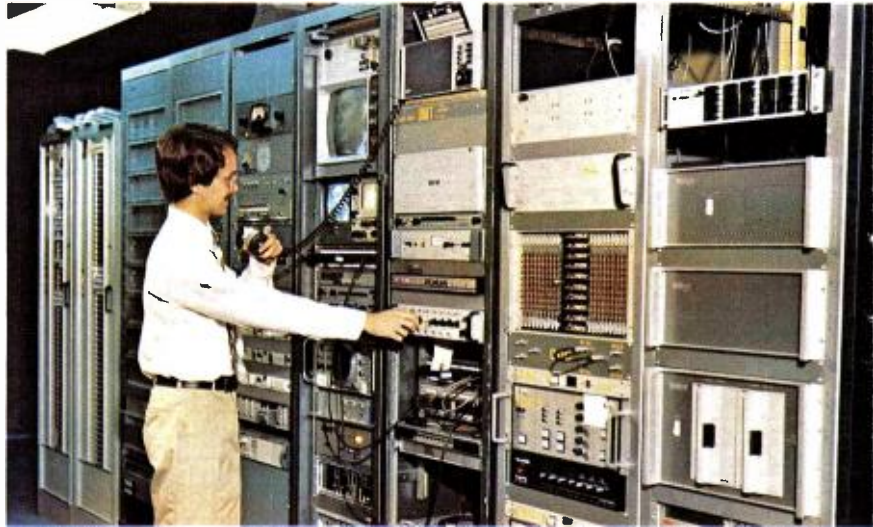
Tactec radio base unit in technical area at studio is used for expediting ENG microwave set-up.
