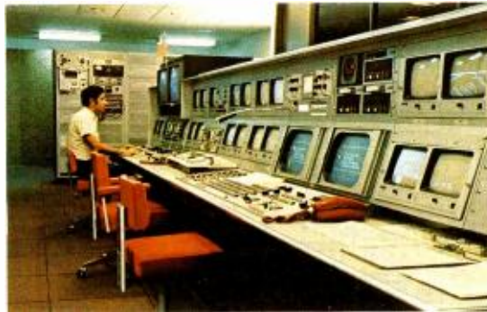
The new technical center for WREG-TV, Memphis, Tenn. is a major customized installation by RCA Systems Engineering (BROADCAST NEWS, Vol. 157).
