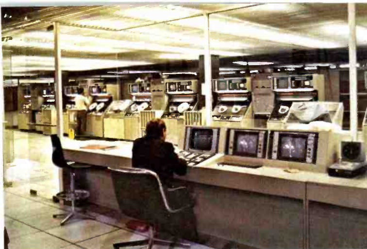
View of video tape area through the window, with tape editing console in foreground.
