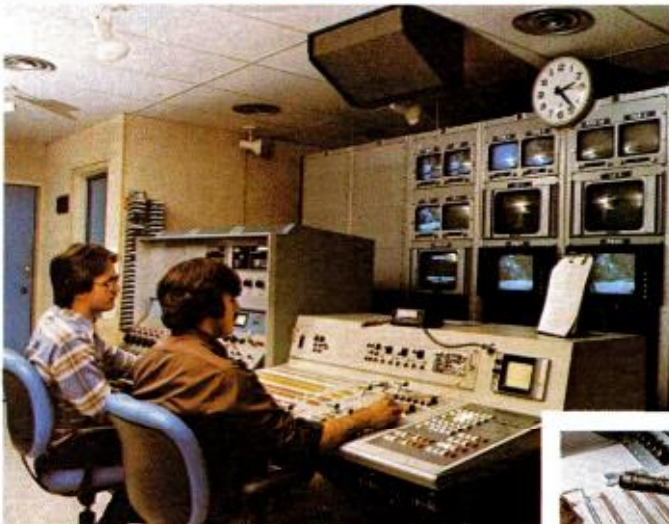
Production Control—clean, functional, attractive.
