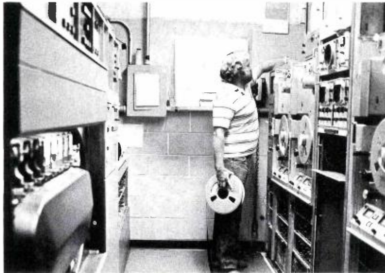
TV-4 Tape Room is compact and well-utilized.
