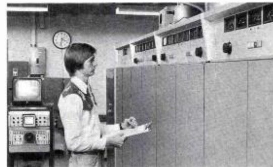
Readings from TTU-60 are logged by staff engineer Terry Snyder.
