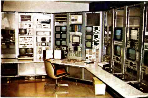
Customized Master Control grouping, with transmitter/STL monitoring facilities on left; switching and machine controls in center, and camera CCU's at right.
