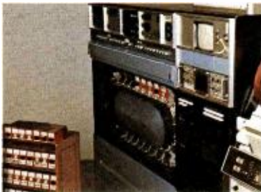
Technical area at CKY includes two TCR-100 video "cart" machines; two-600A VTR's with AE-600 Time Code Editing Systems, and a new TK-28 Telecine system.
