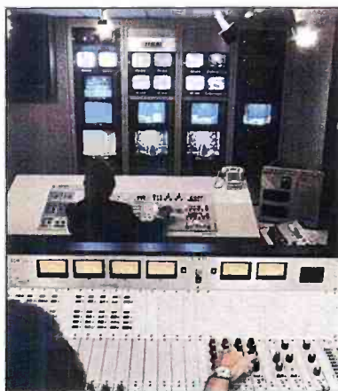
Audio operator has full view of Director Control Room and monitors.
