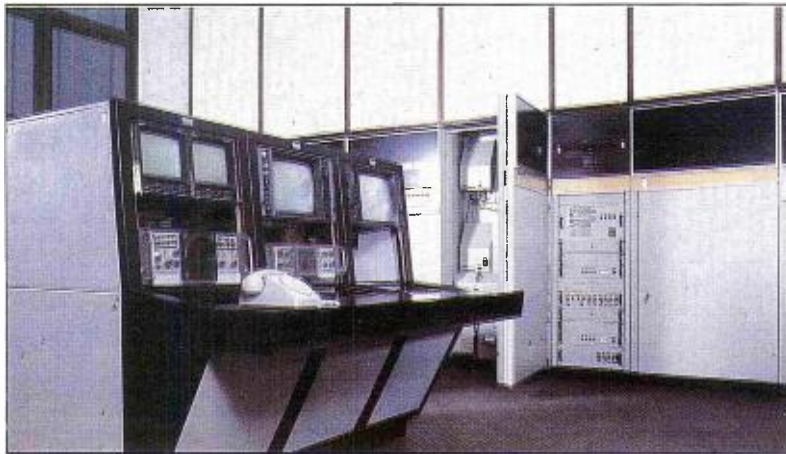
Controls for TTG-30/30L parallel transmitters are console-mounted.
