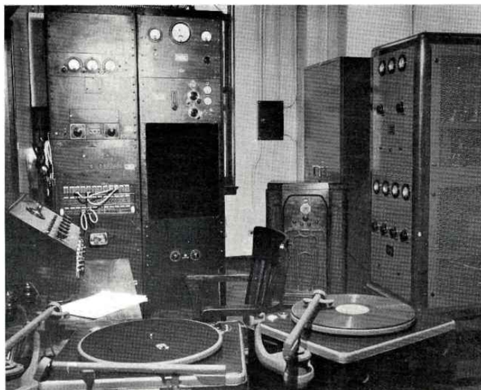
The compact arrangement of the new transmitter and associated equipment for service and efficiency.
