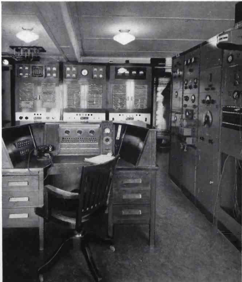
Transmitter house at WBEN, located at Martinsville, N. Y., showing the new 5KW transmitter.
