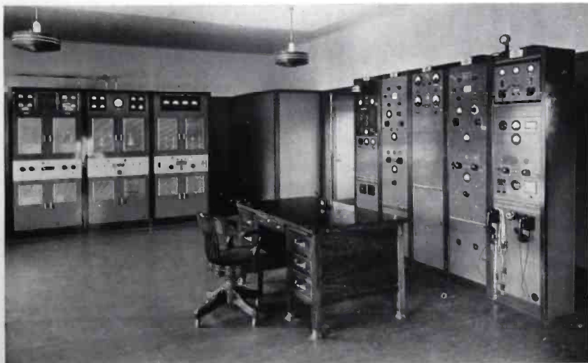
One of the two 5-C Transmitters with studio equipment.
