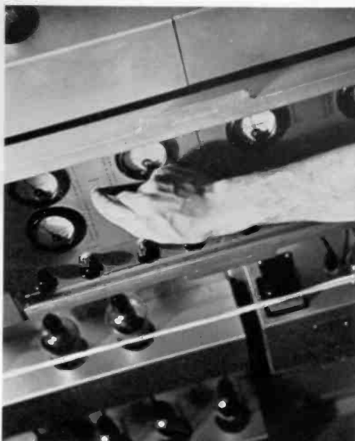
28. A power change switch is useful for changing from 250 to 100 watts for stations operating with reduced power at night. Correct functioning of each device is carefully checked.
