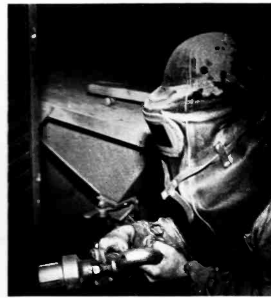
units of the equipment. Sandblasting of frames and panels assures a clean, firm base for lacquer finishes.
