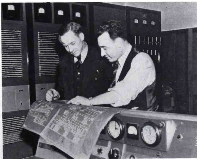
J. A. Chambers, consultant, and C. H. Topmiller, chief engineer, WCKY, conferring during the installation.
