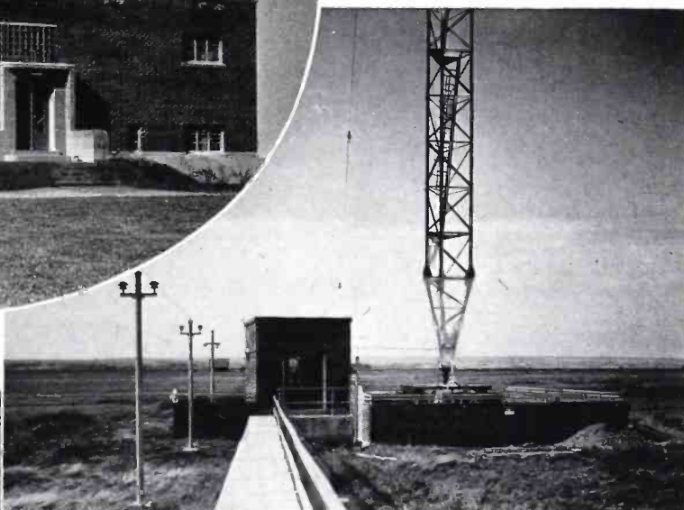
The CBA antenna coupling house and the base of the 460 ft. radiator.
