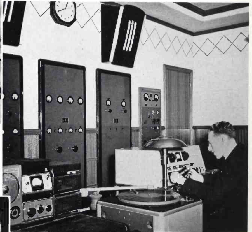
▲ A portion of KFAR's transmitter control. Chief Engr. Stan Bennett at the console. Door to the right gives quick accessibility to RCA 1-G transmitter.
